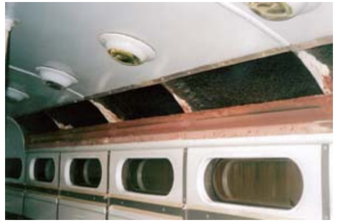
2007 – The interior work was far more than “just a paint job”. Advertising card racks were removed, the steel carlines were cleaned and preserved, and then the card racks were riveted back in place.
