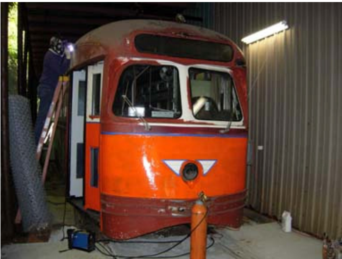
2007 – Progress accelerates as major steel repairs are performed on the roof. Paul Minnick welds in new steel in this photo.
