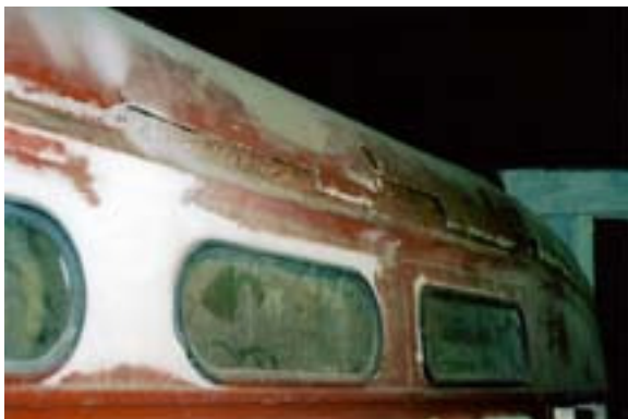
2007 – This shot shows the extent of roof repairs in just one area.
